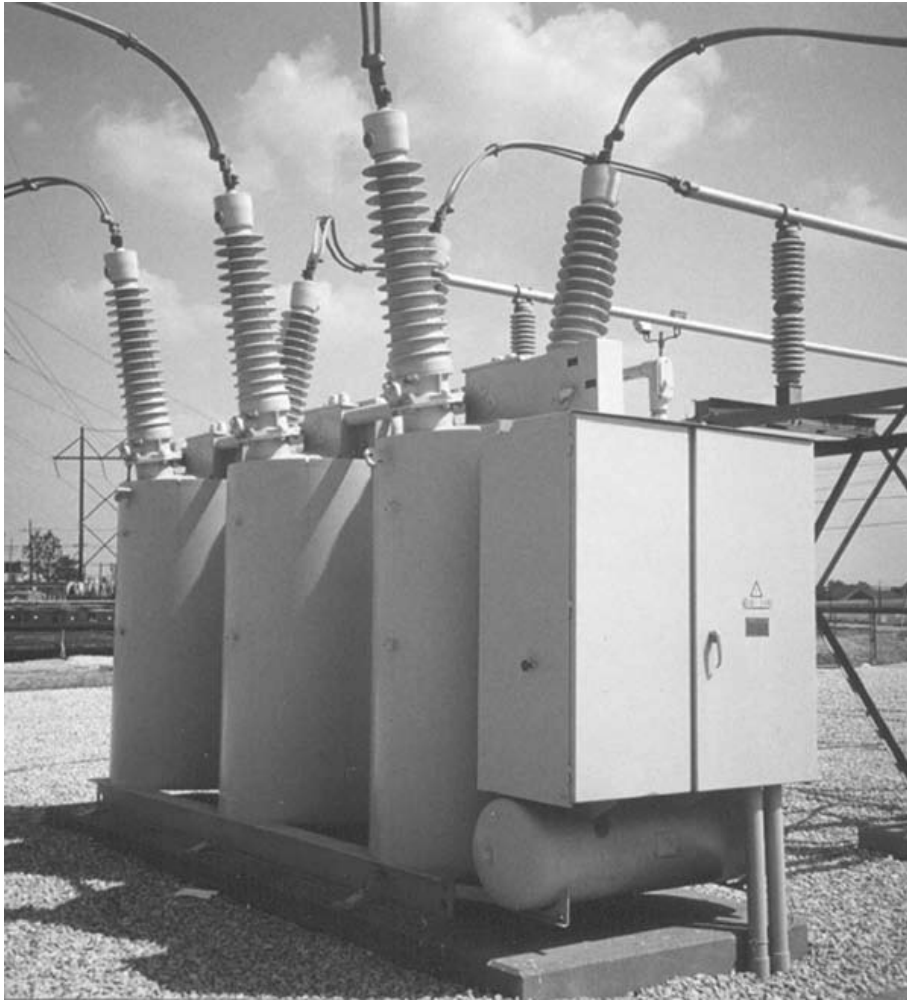
Figure 4-23. Oil circuit breaker.
