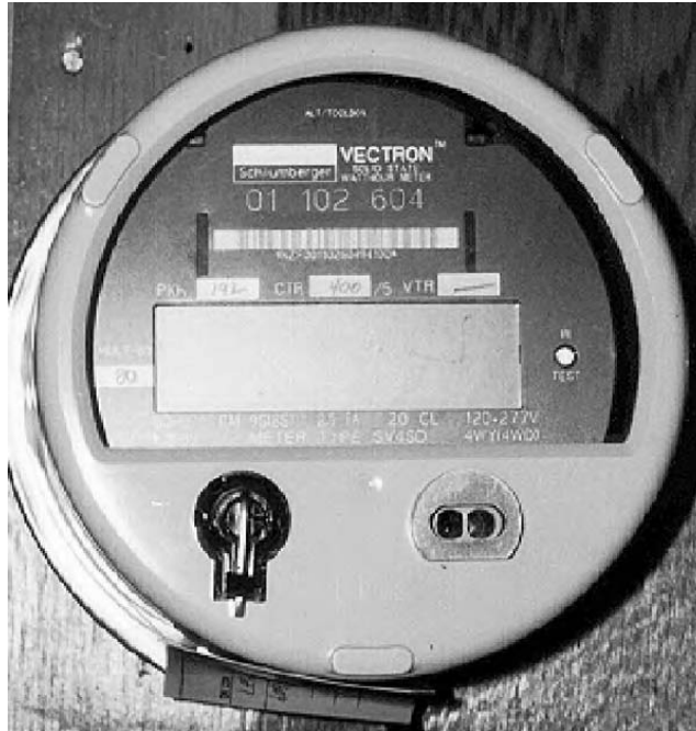
Figure 6-7. Solid-state kWh meter.
