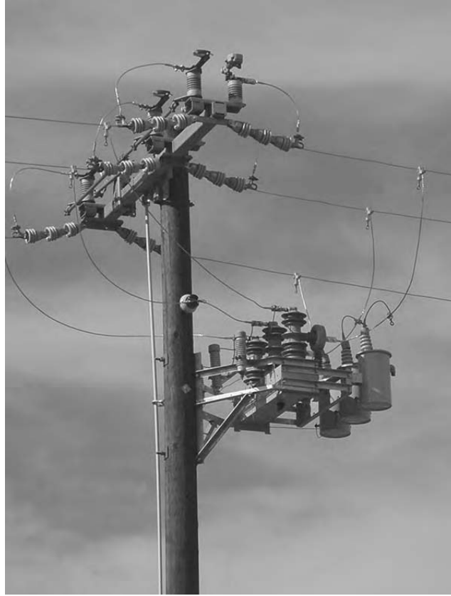
Figure 6-11. Overhead primary metering.
