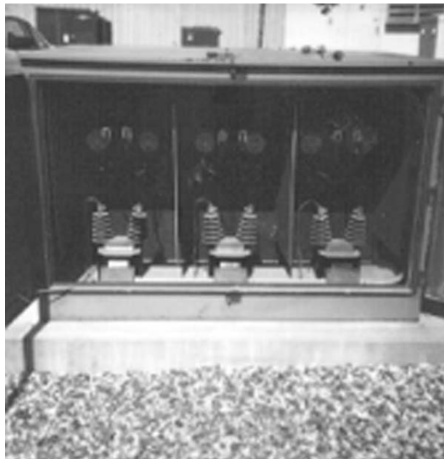
Figure 6-10. Underground primary metering. Courtesy of Alliant Energy.
