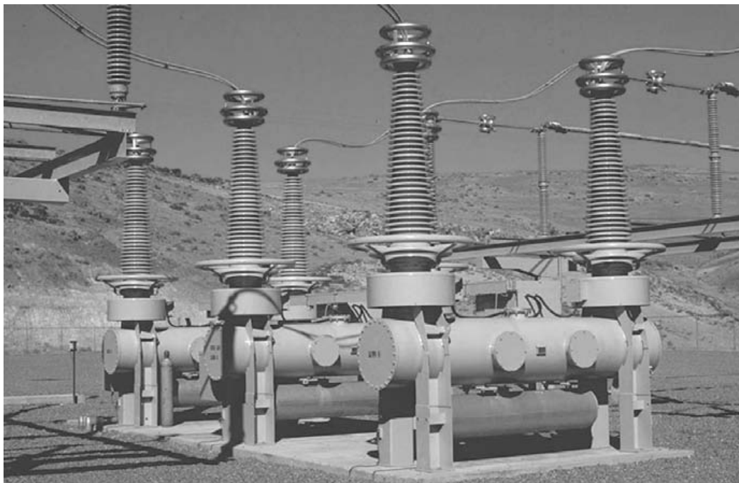
Figure 4-26. 345 kV Gas breaker.
