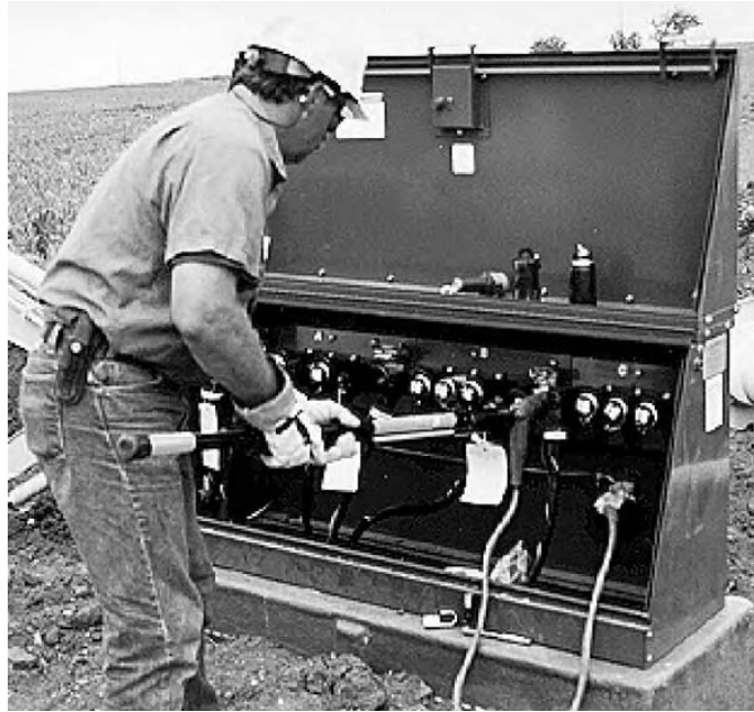
Figure 5-29. Load-break connections. Courtesy of Alliant Energy.
