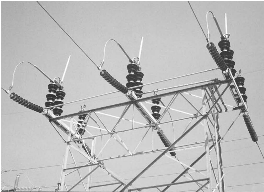
Figure 4-32. Vertical-break switch. Courtesy of Alliant Energy.
