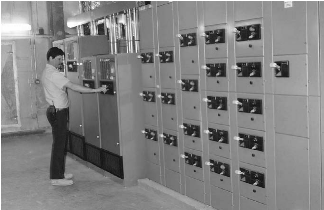
Figure 6-20. Industrial panel. Source: Photovault.
