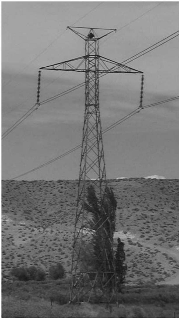
Figure 3-7. Overhead dc transmission line.
