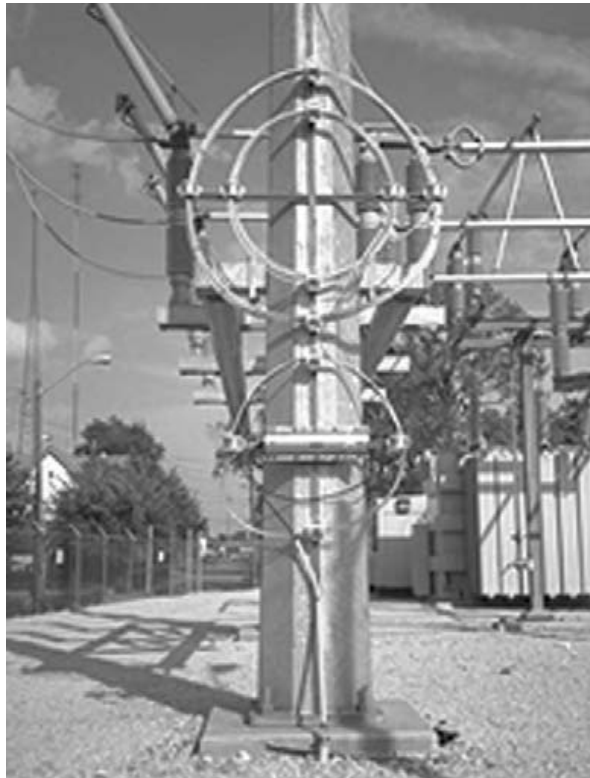
Figure 9-4. Substation fiber optics.
