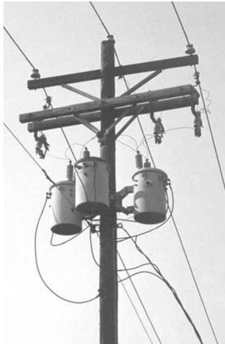
Figure 5-18. Three-phase transformer bank.
