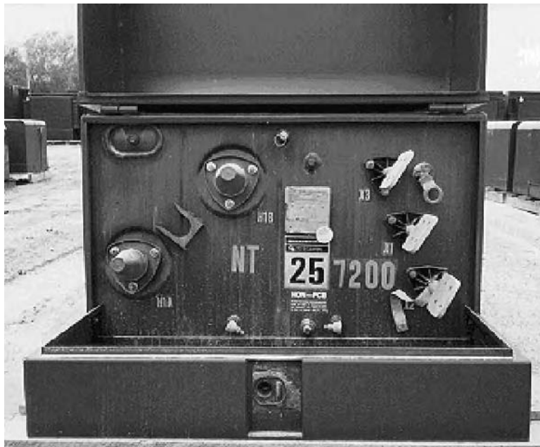
Figure 5-34. Switching transformer. Courtesy of Alliant Energy.
