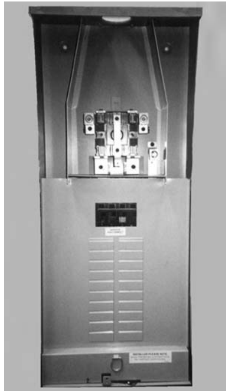
Figure 6-13. Meter cover removed.
