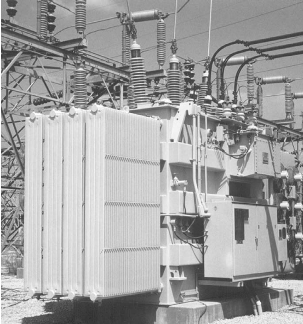
Figure 4-2. Distribution power transformer.
