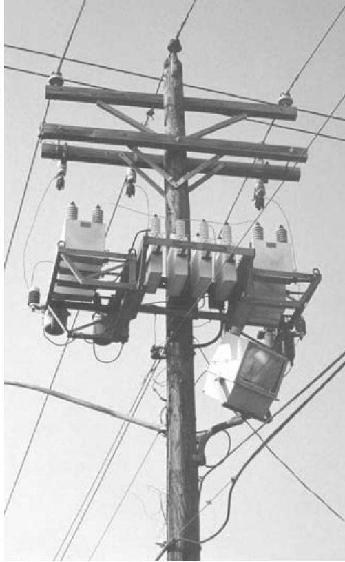
Figure 4-40. Distribution capacitor bank.
